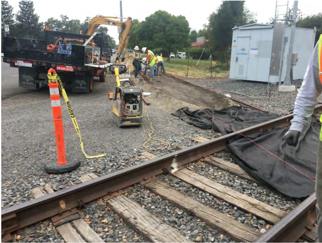
Construction of the sidewalk across the track on the side of Airport Boulevard
