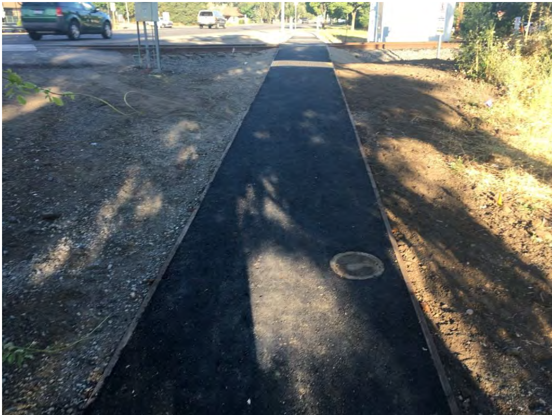
Construction of the sidewalk across the track on the north side of Airport Boulevard
