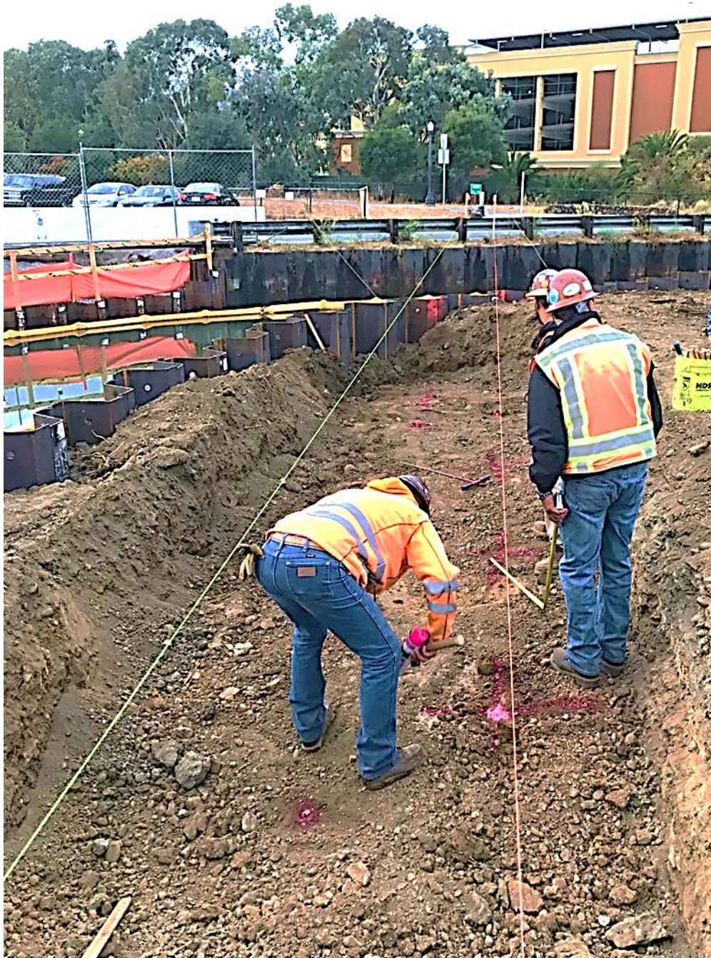
Workers survey placement of the concrete bridge piles at San Rafael Creek Bridge
