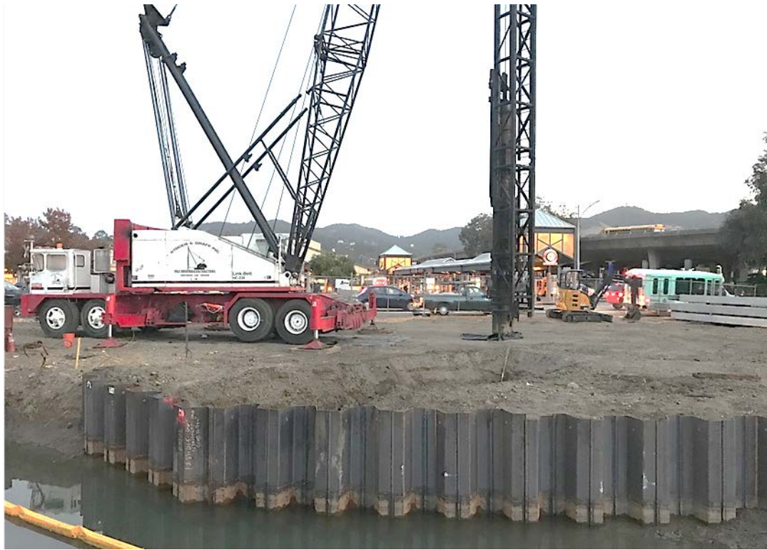
Completed sheet pile installation at the north end of San Rafael Creek Bridge
