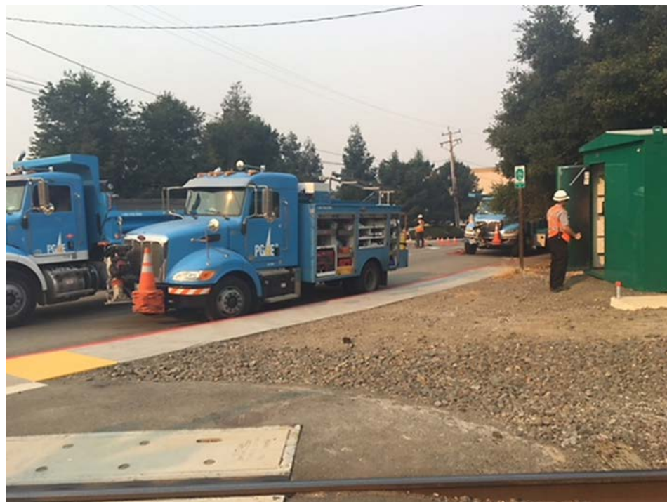
Scene of a PG&E gas line break in San Rafael
