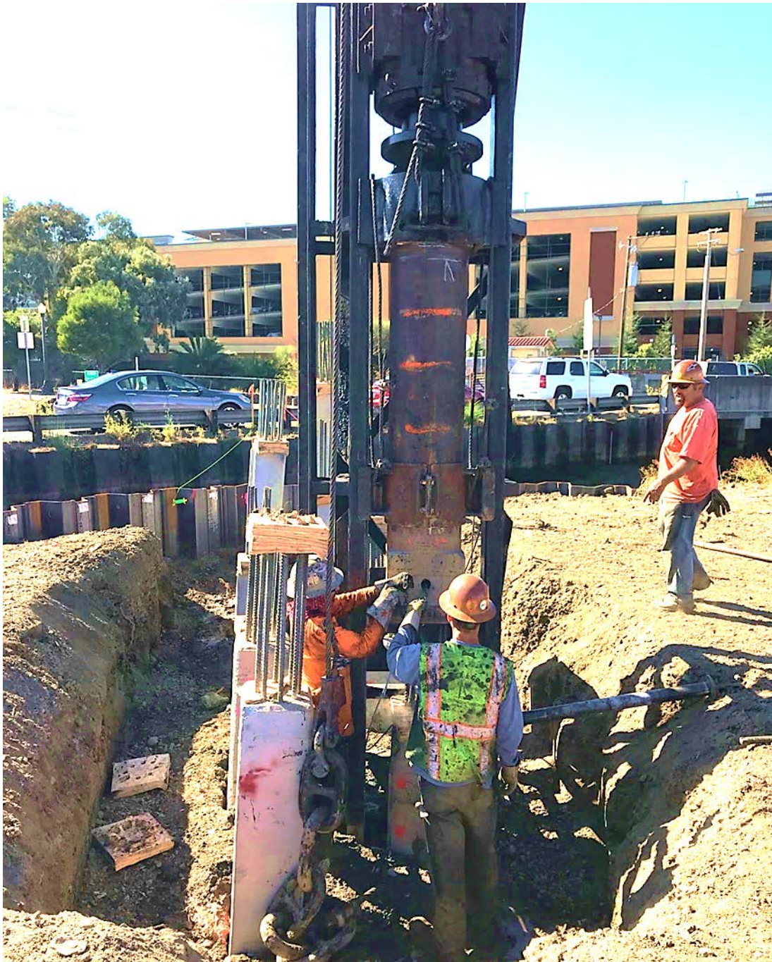
Crews begin pile driving the concrete piles at the San Rafael Creek Bridge
