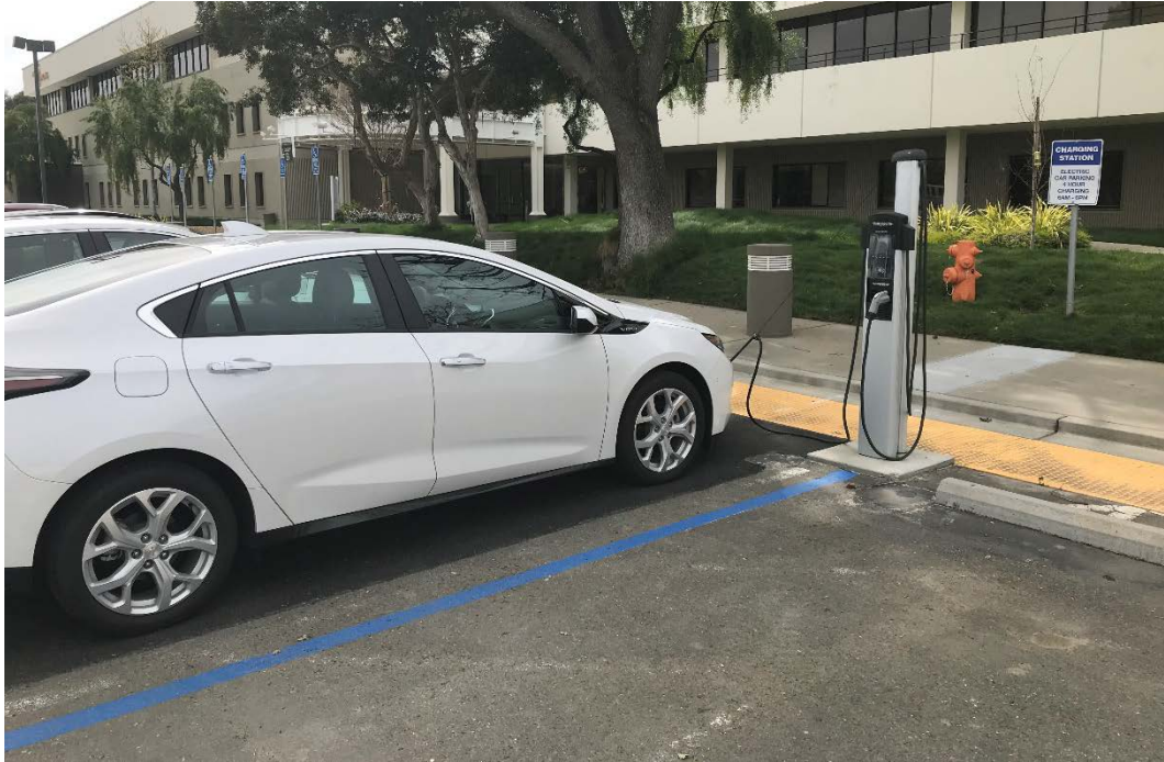
Workplace Public Charging Station at MarinCommons
