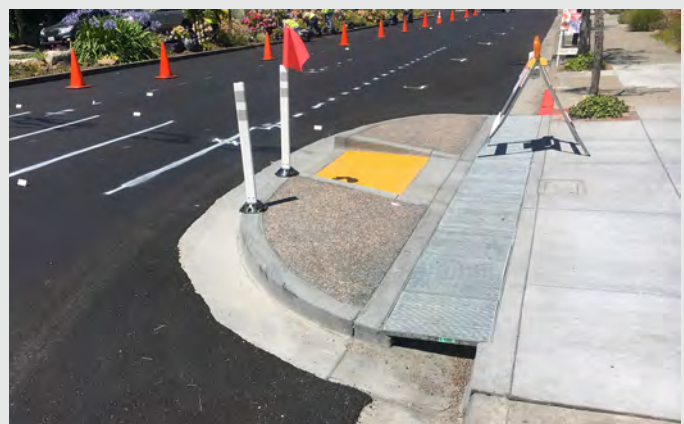
Curb extensions , sometimes called bulb-outs, make pedestrians more visible to drivers while providing additional room to wait before crossing the street. The extensions also reduce crosswalk lengths and slow turning vehicles.
