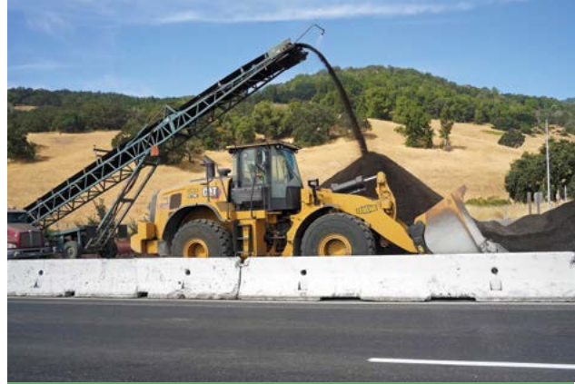
Construction is making great progress on the final section of HOV Lanes!
